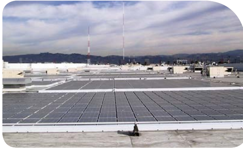
Rooftop solar panels
