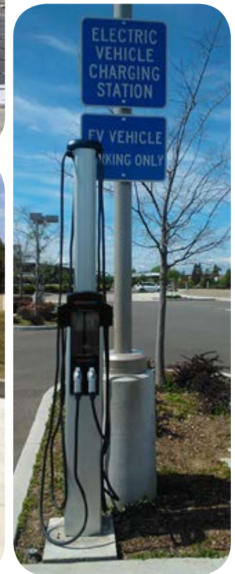
Electric vehicle charging station
